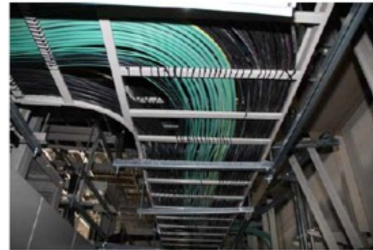
Electric Wiring Room
