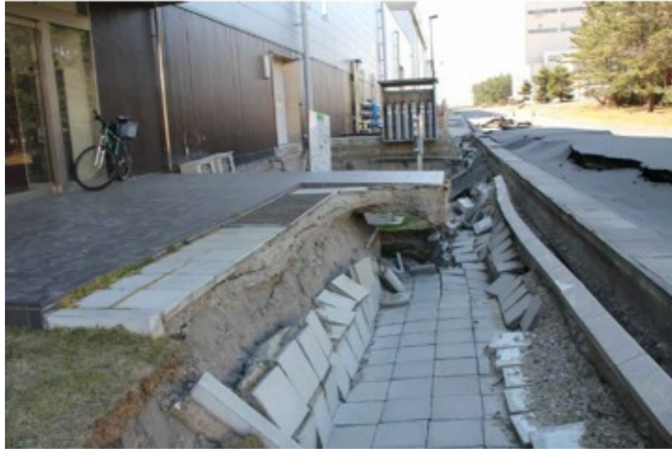
About 1.5 m drop as seen above, over a wide area. Electric wires and water pipes were all damaged.
