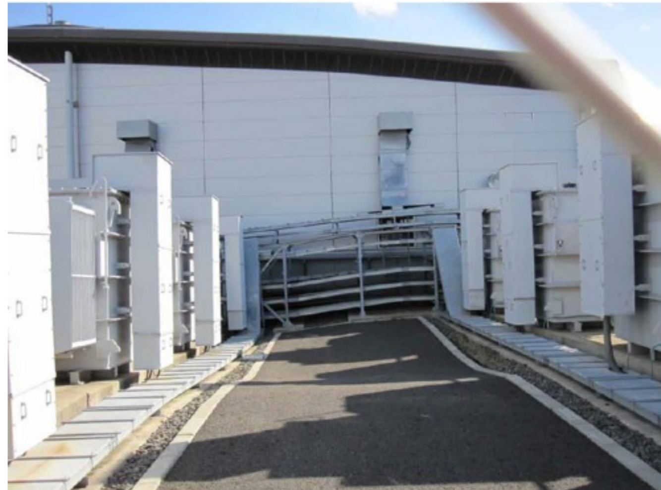
Cable racks were all bent.
