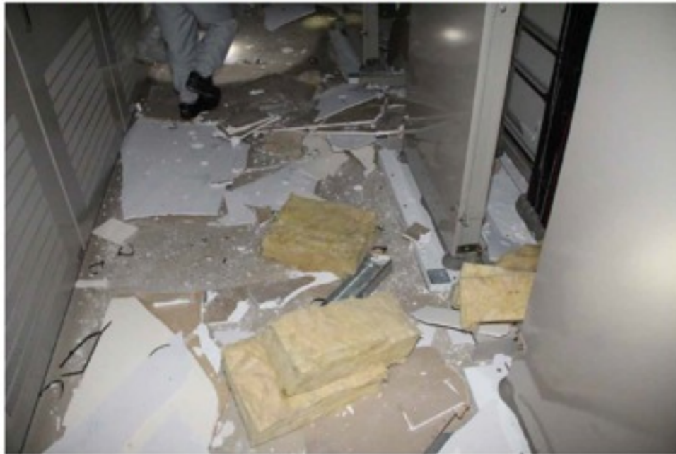
Side buildings were severely damaged (due to less number of underpins), whereas central area for Linac had no damages including klystrons. 5
