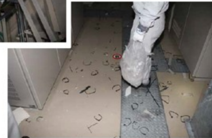
Cable Rack (upper) and many bundles were scattered on the floor below the cable rack (lower).
