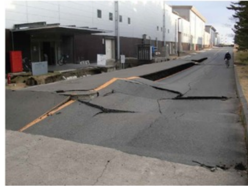
Serious cracks on the road. This is a typical one and can be seen all over the J-PARC area.
